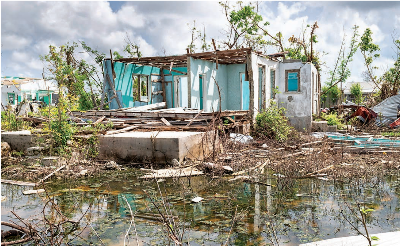
The aftermath of Hurricane Irma in Codrington, Barbuda (September 2017) Photo: UN/Rick Bajornas
